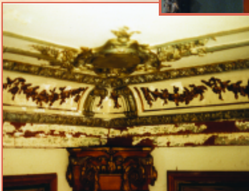
Plaster elements decayed due to moisture infiltration.
